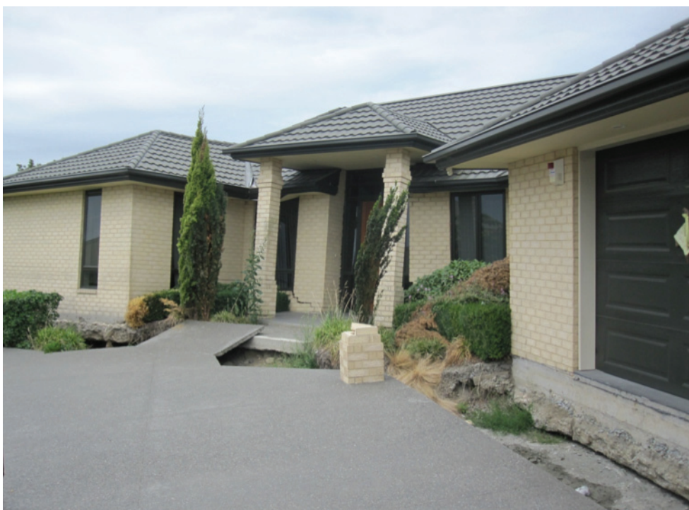
Figure 5. Typical liquefaction damage to modern single-family home in Christchurch, New Zealand. Note that this home will likely need to be completely rebuilt due to extensive foundation damage.
